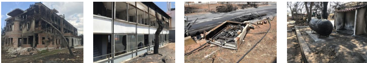
Figure 13. Some examples of latent risks inside a WUI area after the pass of fire include unstable buildings, broken and falling glazing, laying electrical installations or damaged LPG tanks among others.
